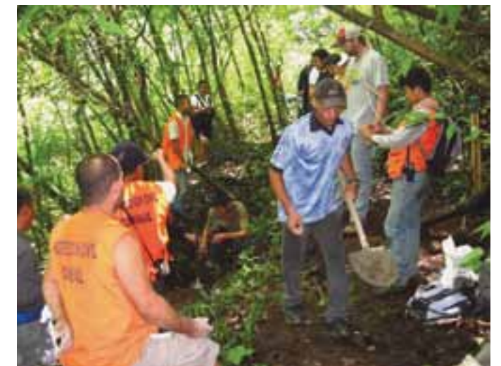
Informal concrete benchmarks are installed to monitor slope movements at a surface crack following Tropical Depression 12E, November 2011.
