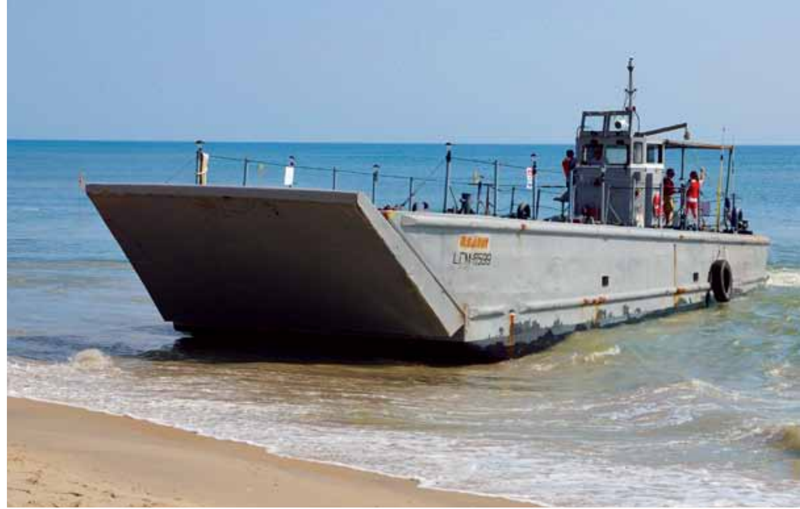
Elgar and his team clear a 100 meter long by 30 meter wide trench with a Vietnam War-era military landing craft.
