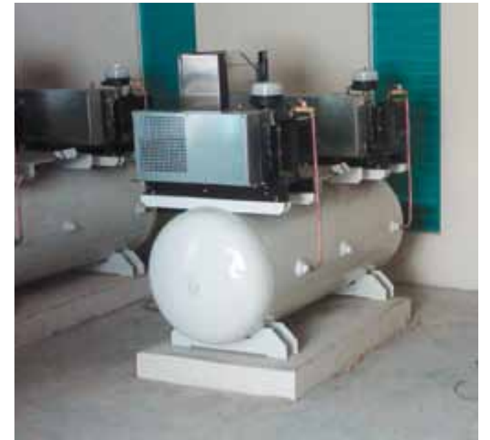
The 10 HP compressors above pump air into the diffusers located at the bottom of lake Toa Vaca, moving around 150,000 gpm.
