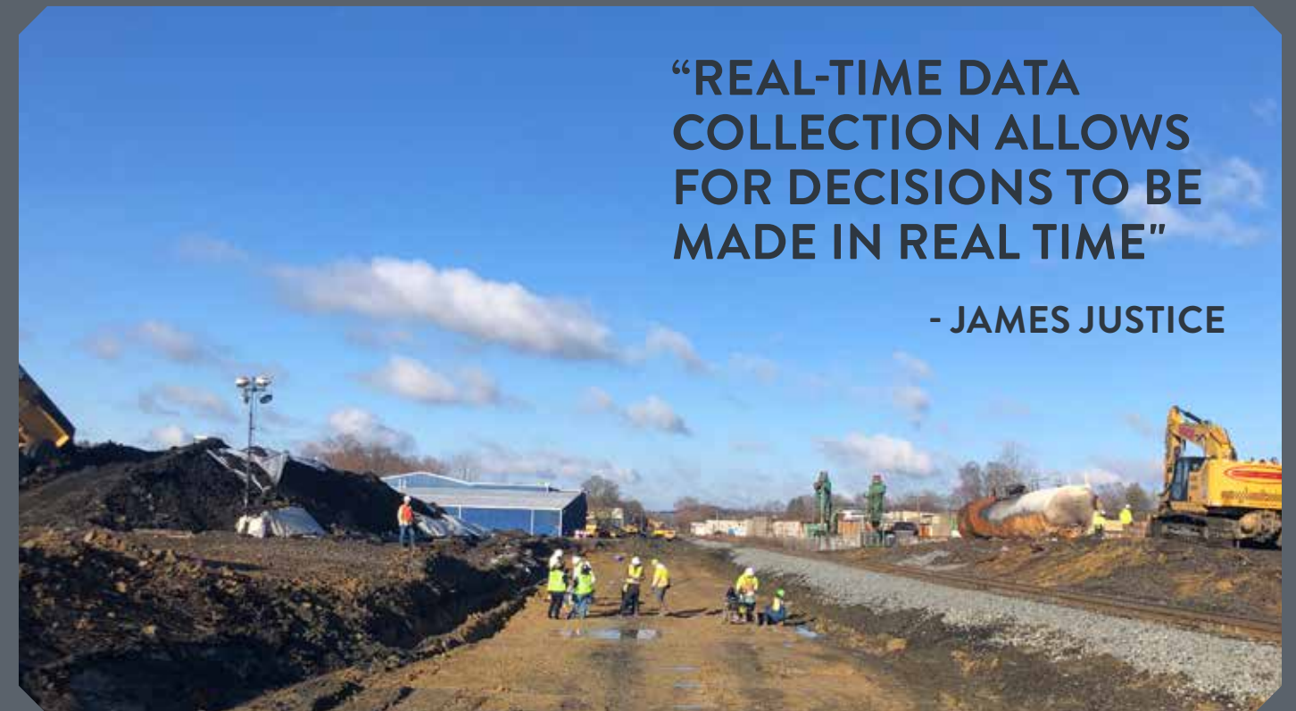
(Right) Norfolk Southern and EPA conducting soil sampling beneath the excavated rail track area.
